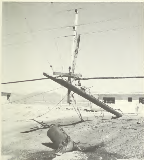
Figure 5.105. Transformer fallen from collapsed utility pole (5 psi peak overpressure), Nevada Test Site.
