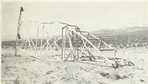
Figure 5.102a. Collapsed suspension tower (5 psi peak overpressure, 0.6 psi dynamic pressure from 30-kiloton explosion), Nevada Test Site.
