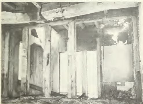
Figure 5.20a. Upper photo: Reinforced-concrete, aseismic structure; window fire shutters were blown in by blast and the interior gutted by fire (0.12 mile from ground zero at Hiroshima). Lower photo: Burned out interior of similar structure.
