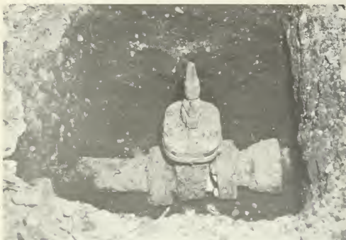
Figure 5.106a. Four-inch gate valve in water main broken by debris from brick wall (0.23 mile from ground zero at Hiroshima).
