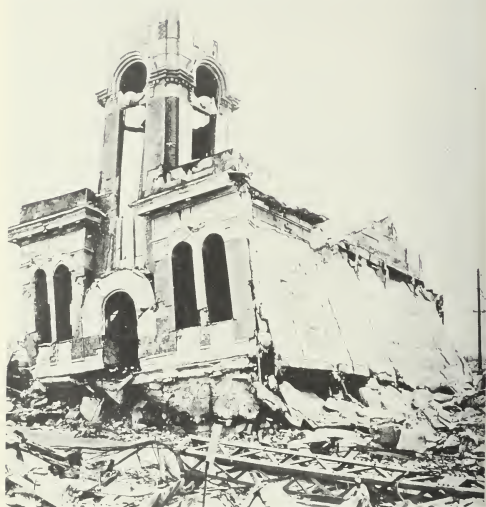
Figure 5.26. Two-story, steel-frame building with 7-inch reinforced-concrete wall panels (0.40 mile from ground zero at Hiroshima). The first story columns buckled away from ground zero dropping the second story to the ground.
