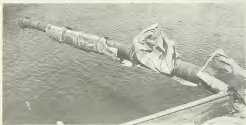
Figure 5.106b. Broken portion of 16-inch water main carried on bridge (0.23 mile from ground zero at Hiroshima).
