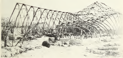
Figure 5.29. Single-story, light steel-frame building (0.80 mile from ground zero at Hiroshima); partially damaged by blast and further collapsed by subsequent fire.
