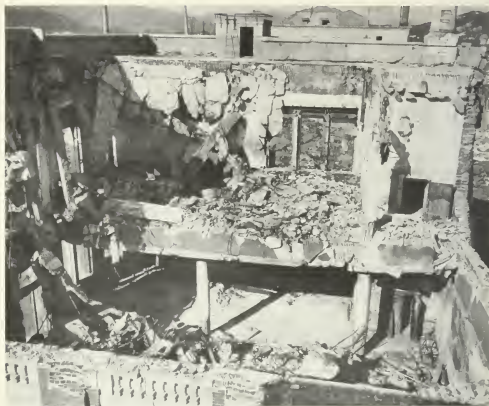
Figure 5.23. Reinforced-concrete building showing collapsed roof and floor slabs (0.1 mile from ground zero at Nagasaki).
